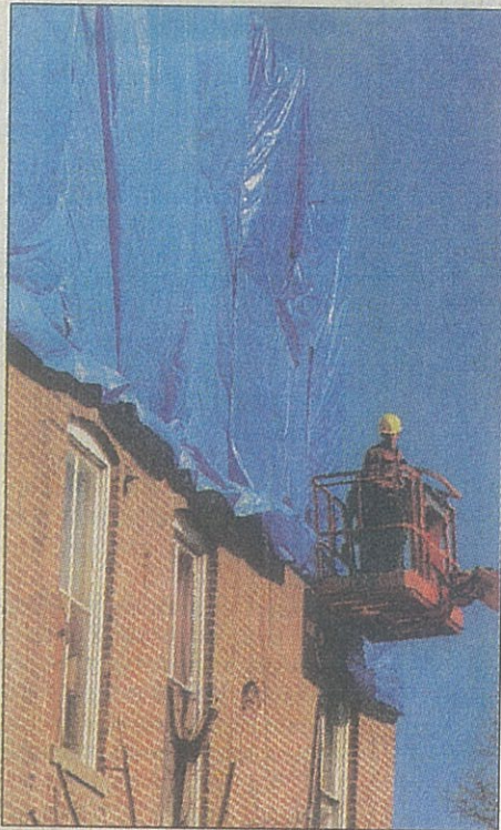
Workers use a lift crane to fasten tarps on a Clarksville building. The owner says the city damaged it unnecessarily.
